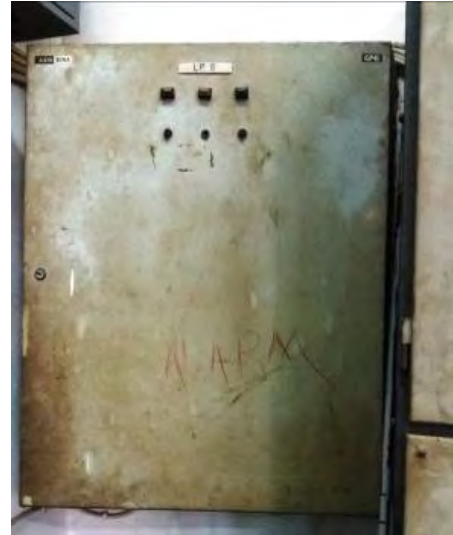
Gambar 10. Cover panel utama di bengkel listrik
