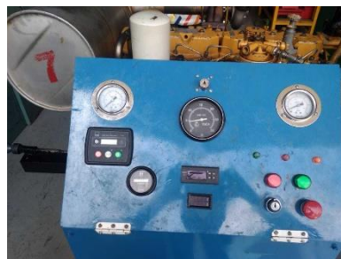
Figure 2. Control Panel of Engine 3066
