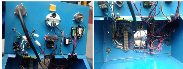
Figure 5. Visual state of the cables on the control panel
