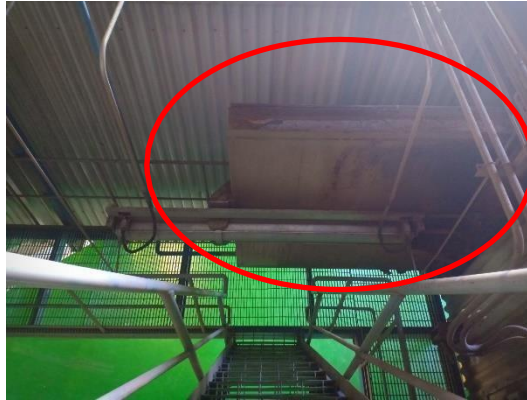
Gambar 2. Shut Off Damper Hot PA
