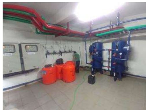
Figure 2. Injection of Chlorine
