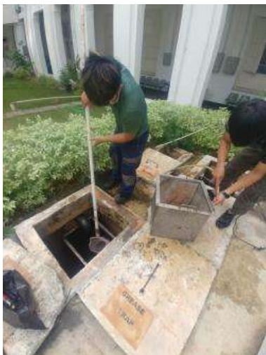
Figure 4. Cleaning Process in Grit Chamber
