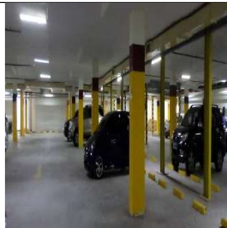
Figure 2. The decrease in almost every basement column, even reaching 189 mm (based on surveyor measurements)
