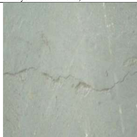
Figure 4. The floor has decreased (new cracks have returned to old cracks)
