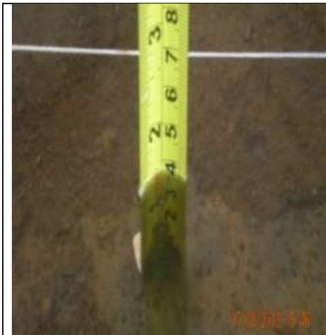
Figure 1. Basement / Plate Structure: broken and deflated 7cm
