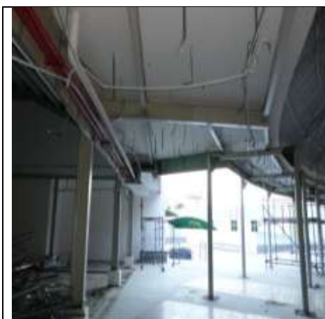
Figure 5. The beam is tilted and bent
